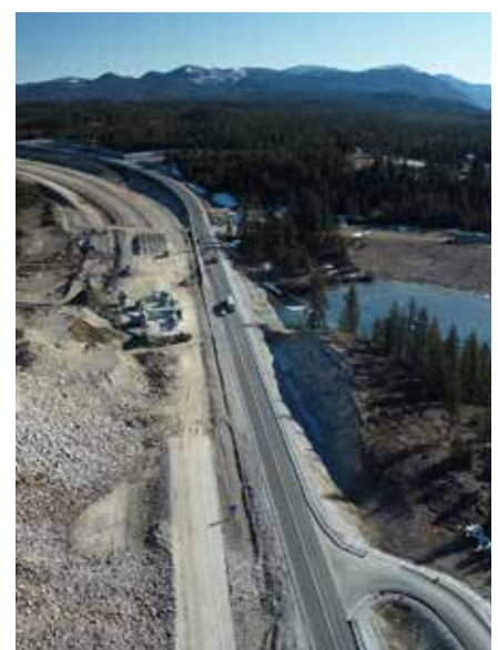
Blasted material was crushed and used on the project for rock lined ditches, roadway base, and rip rap.
